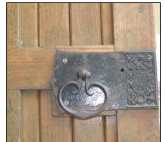
Historic door hardware, like at Jackson Memorial Hall, should be carefully maintained.
