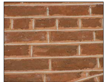
Brick, one of the most common building materials on Post, can be seen at 450 Institution Hill.
