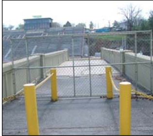
The pedestrian bridge is suffering from structural cracks and settling – creating unsafe conditions for pedestrians.
