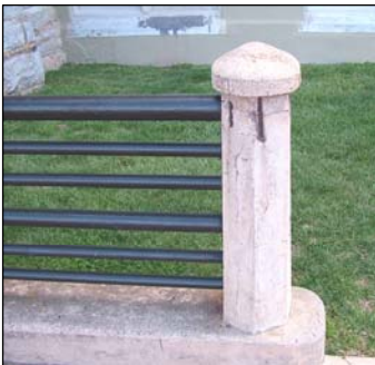
Existing concrete bollards are generally in poor condition.
