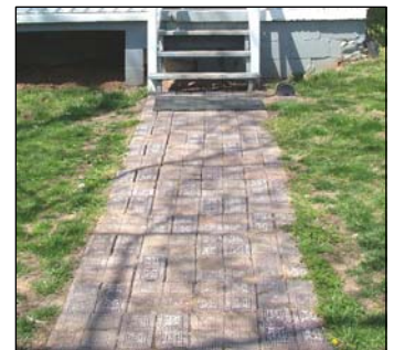
Lexington Brick sidewalks, like this one at 307 Letcher Avenue, are a character-defining feature on the Post.
