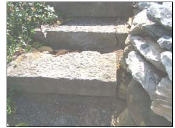
Stairs at 406 VMI Parade are cracking and spalling.
