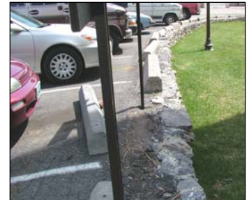
Asphalt parking in front of Scott Shipp Hall has concrete wheel stops atop a deteriorating stone retaining wall.
