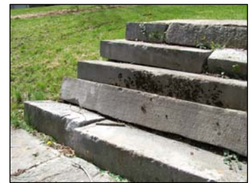
Cut limestone steps provide access to the terraces at Stono but are in poor condition.
