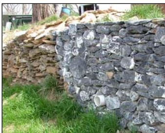
Replacement walls are not consistent with historic walls in color and materials.
