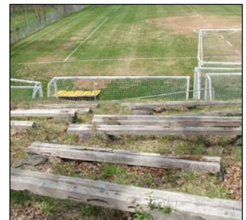
Wooden bleachers overlooking the lacrosse field are in poor condition due to settlement and decay.
