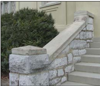
The use of stone is often seen in small-scale building features, such as this railing at Maury-Brooke Hall.
