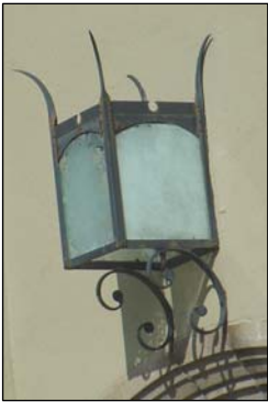
Metal light fixture on the Barracks, above, and at 410 VMI Parade, below.
