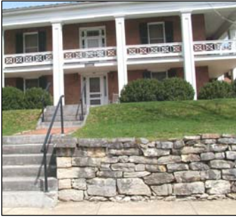
The existing stone retaining wall in front of the Post Hospital retains historic integrity.
