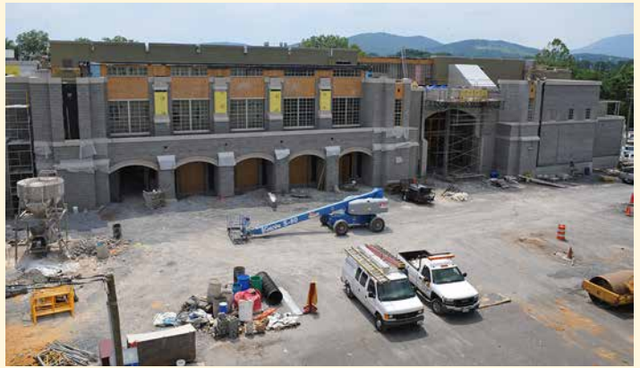
The construction of Marshall Hall and the courtyard progress in June 2008.—VMI File Photo by Kevin Remington.
