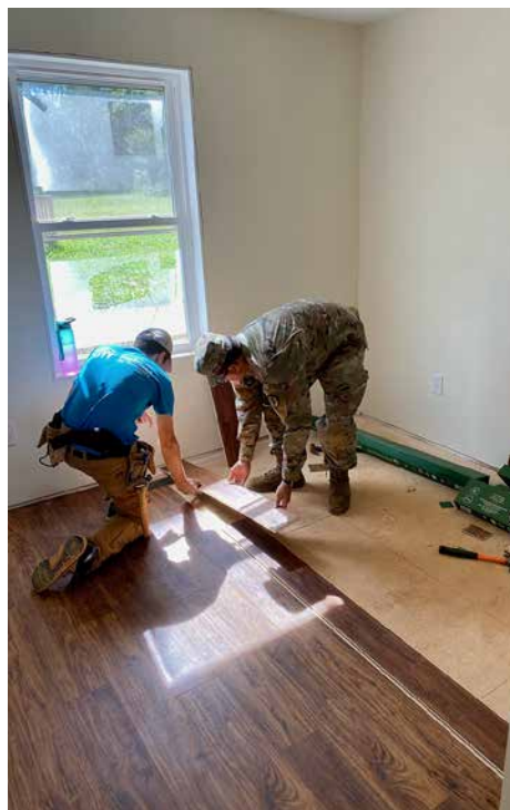
Suttipat Muangna '24 lays floorboards with a Habitat employee on a build site earlier this semester. —Photo courtesy of Col. Valentina Dimitrova-Grajzl.
